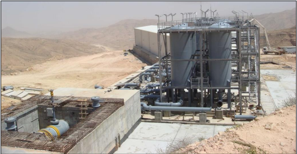
Valve Structure, Surge Vessels – Pump Station
