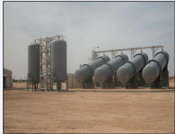
Outlet Surge Vessels
