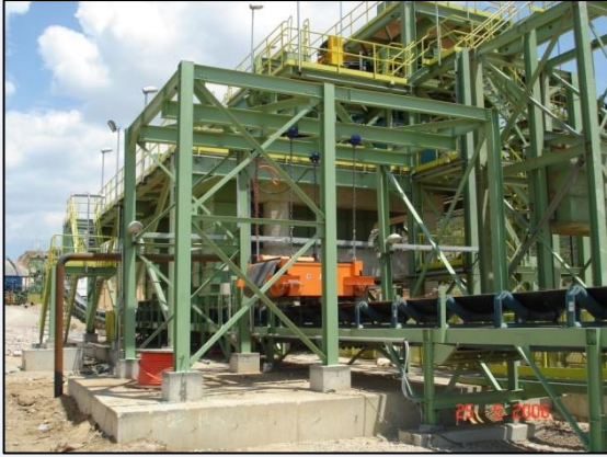
Secondary & Tertiary Crusher
