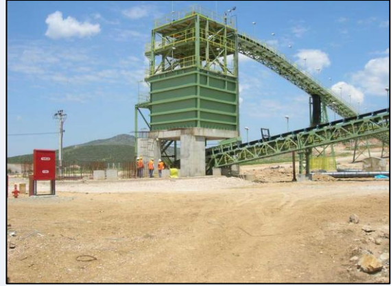
Secondary & Tertiary Crusher
