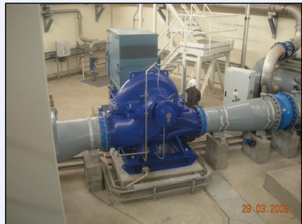
Pump and Motor Set
